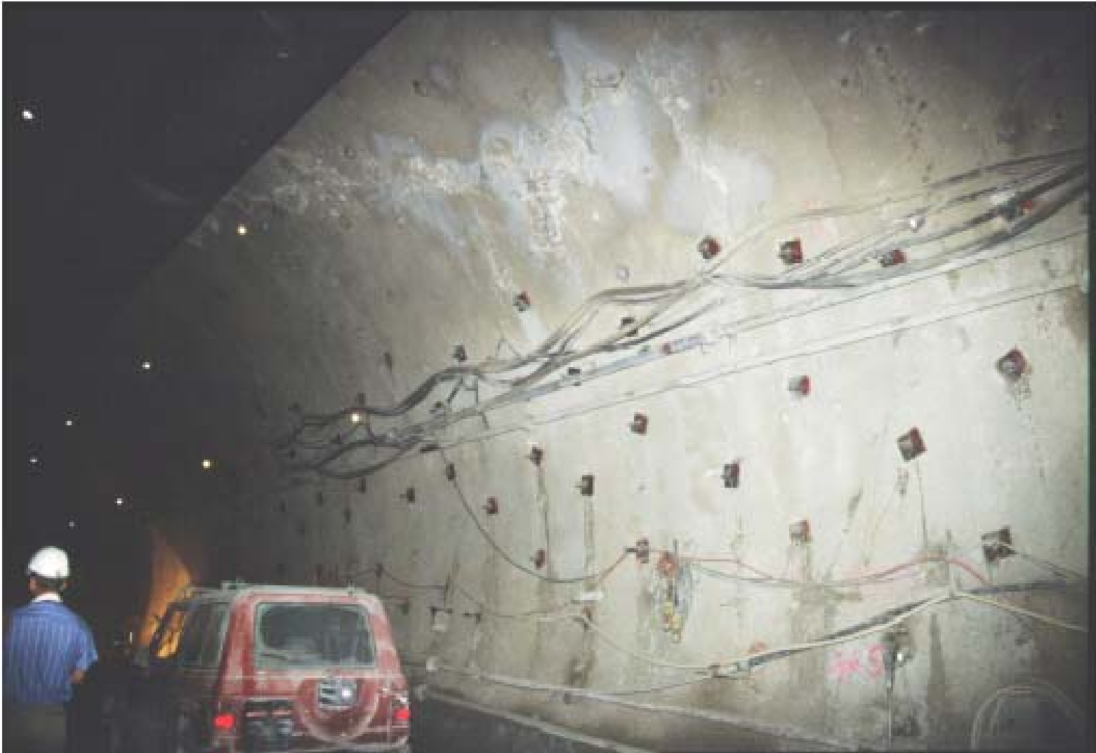
Figure 8. Damage to the tunnel lining due to the anisotropic deformations between stations 1785 and 1800.
